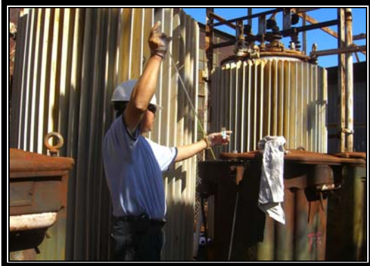
- Transformer Oil Sampling -
